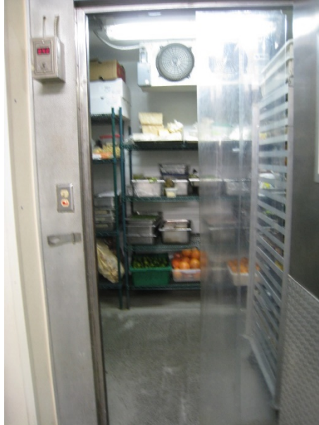
Figure 3-4. Strip Curtain at Site 10
