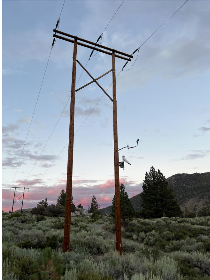
SCE Transmission, June Lake CA
