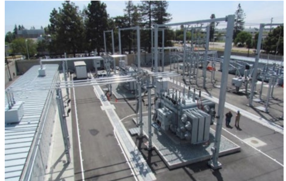
Distribution and Customer Substations
